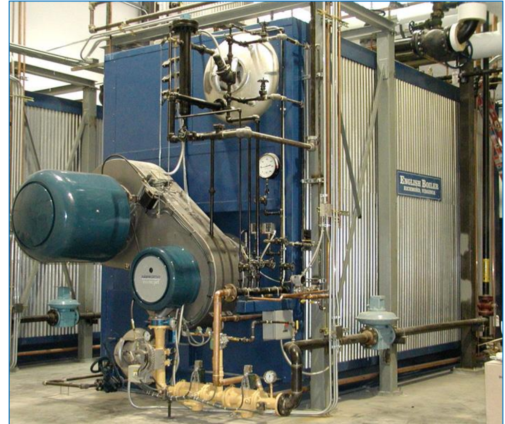
D-Type packaged watertube boiler Courtesy English Boiler Inc.
